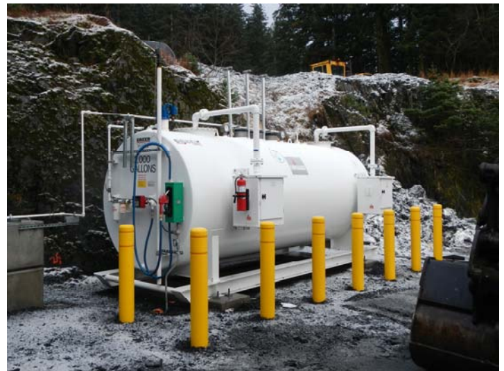
Baler Building Fuel Tank
